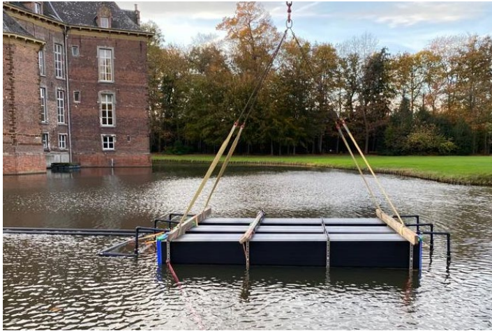
Heat exchanger in the water
